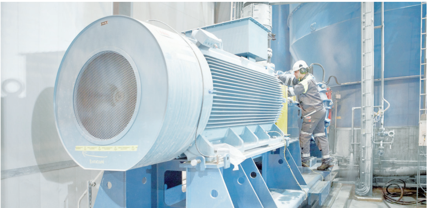
Object metering is used to show the electricity consumption where it occurs
